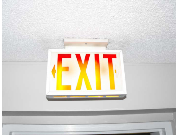
Illustration 11: Emergency exit sign
