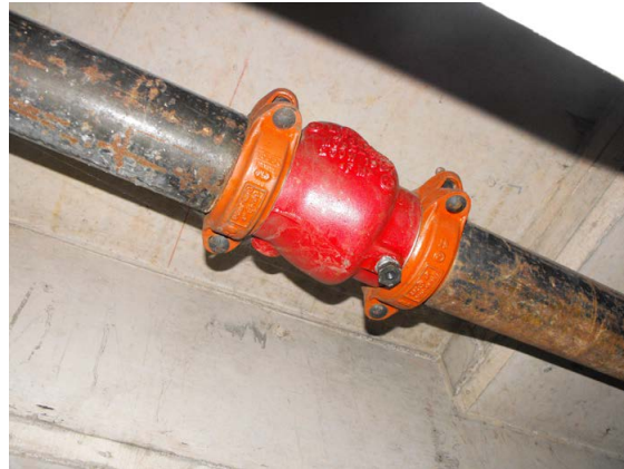
Illustration 8: Four inch check valve for fire department connection (In locker #43 in Garage)
