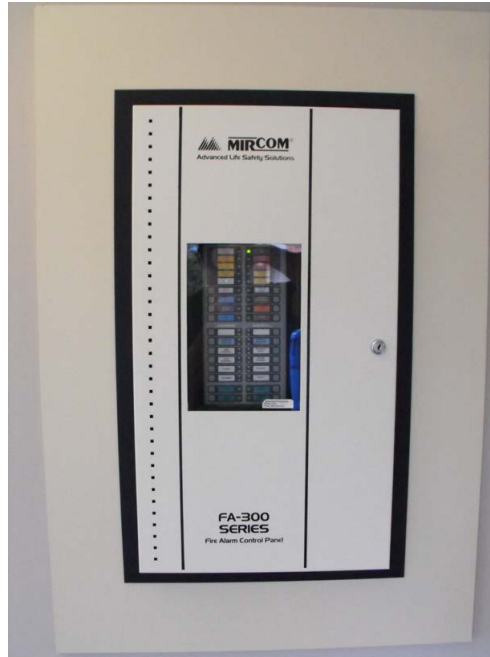
Illustration 1: Fire Alarm Panel located in outer lobby
