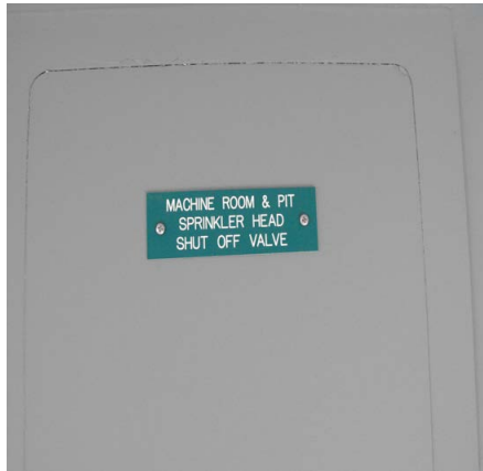
Illustration 15: Machine room and pit sprinkler head shut off valve
