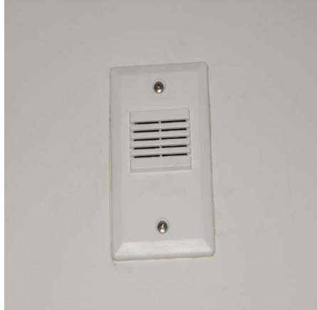
Illustration 6: Fire alarm in residents units
